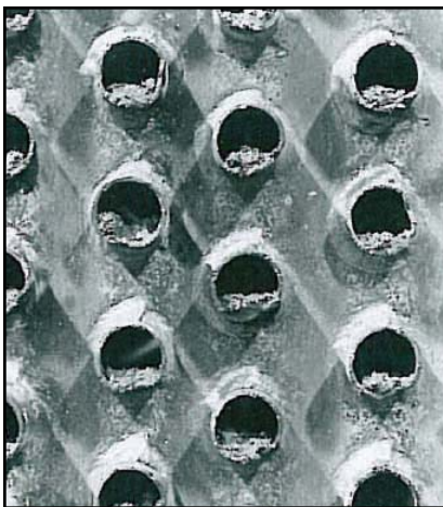
Picture #2 - Fouling of Chiller Condenser Tubes
