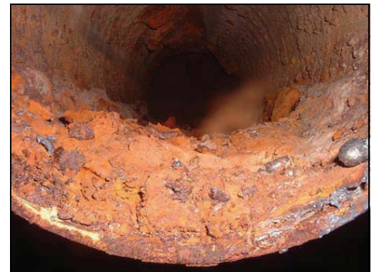
Picture #1- Interior Pipe Deposits
